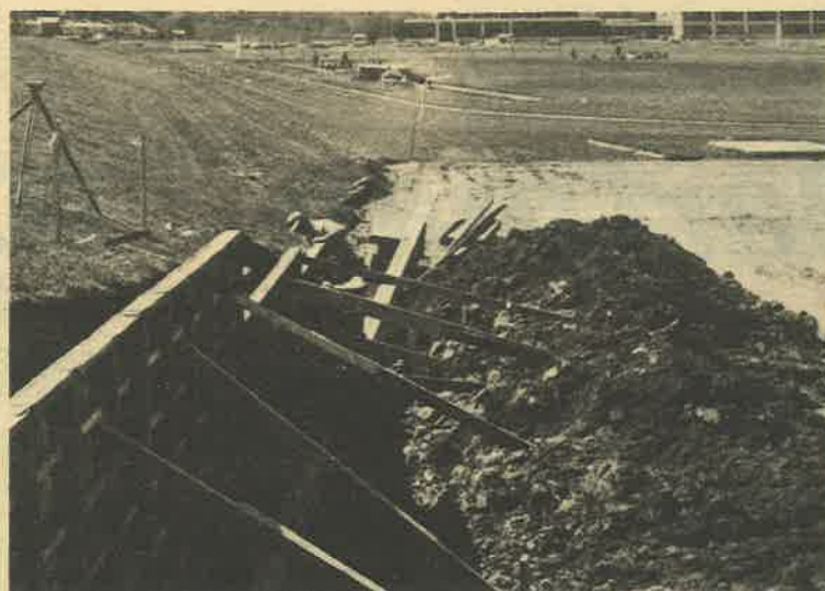
The construction of the new tennis courts at the senior high is now underway. They are expected to be completed early this summer.
