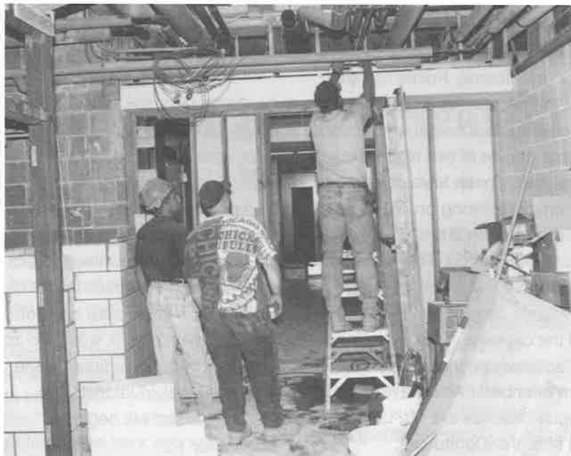
Construction is still in progress from the last referendum. The science lab remodeling is complete and students are now able to have classes there.
