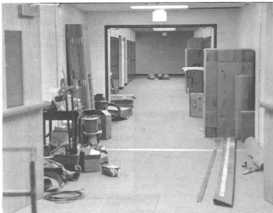
When this picture was taken this section of the new wing was not quite finished.
